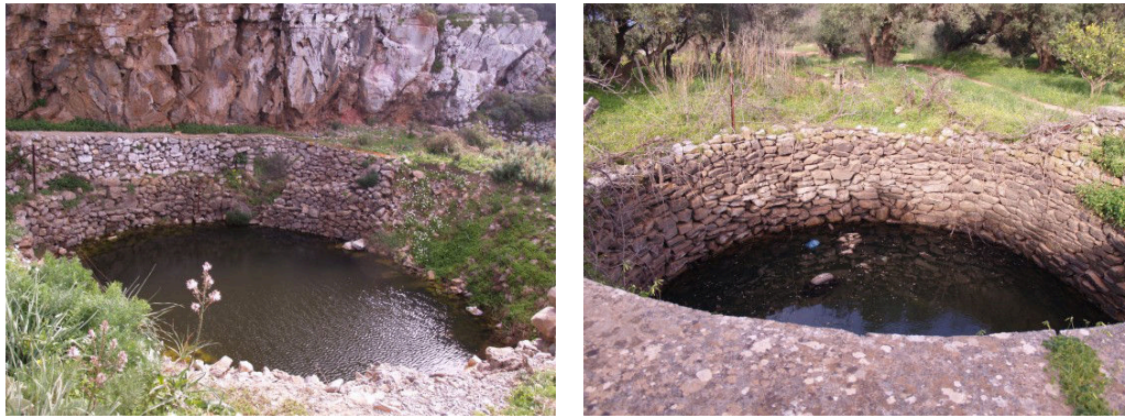
(a) Large cistern in Dilakko, where a large section of the wall is collapsed.
